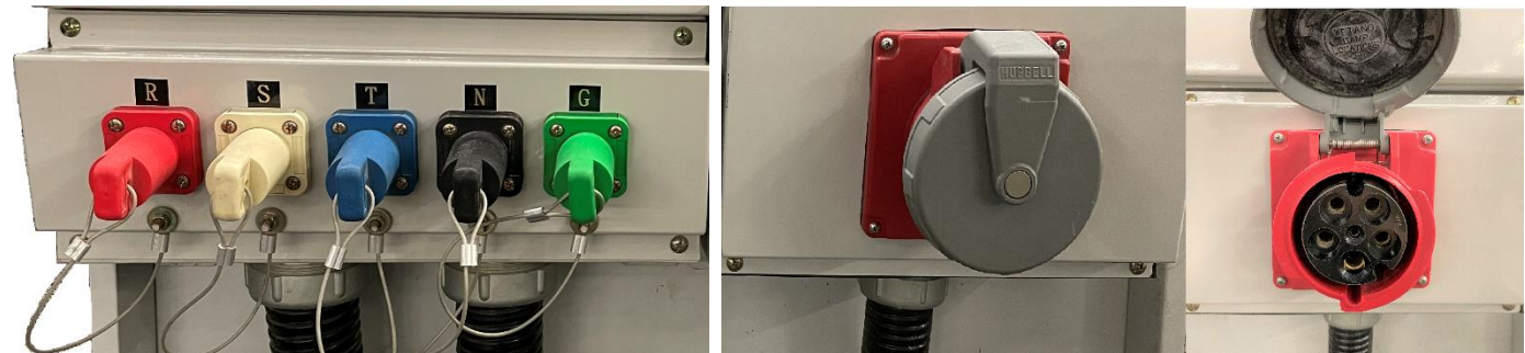
Figure 3.7.1- Additional Power Supply
