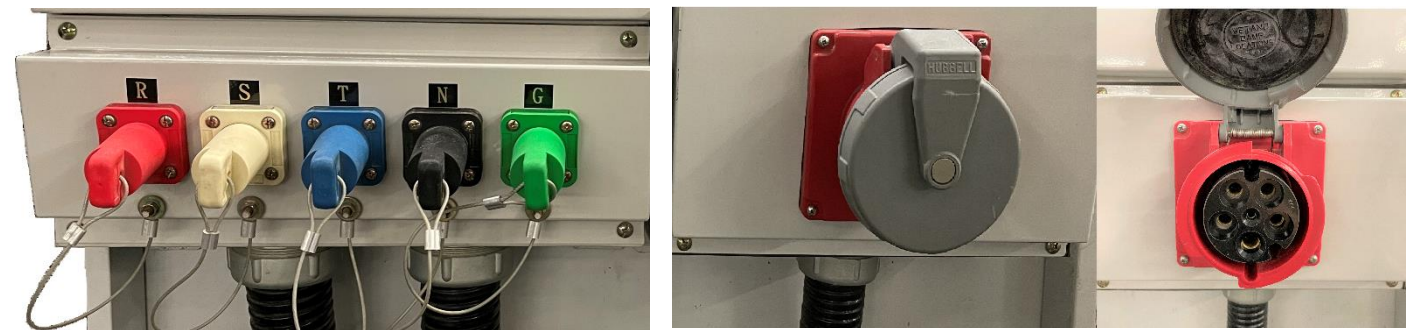
Figure 3.6- Additional Power Supply
