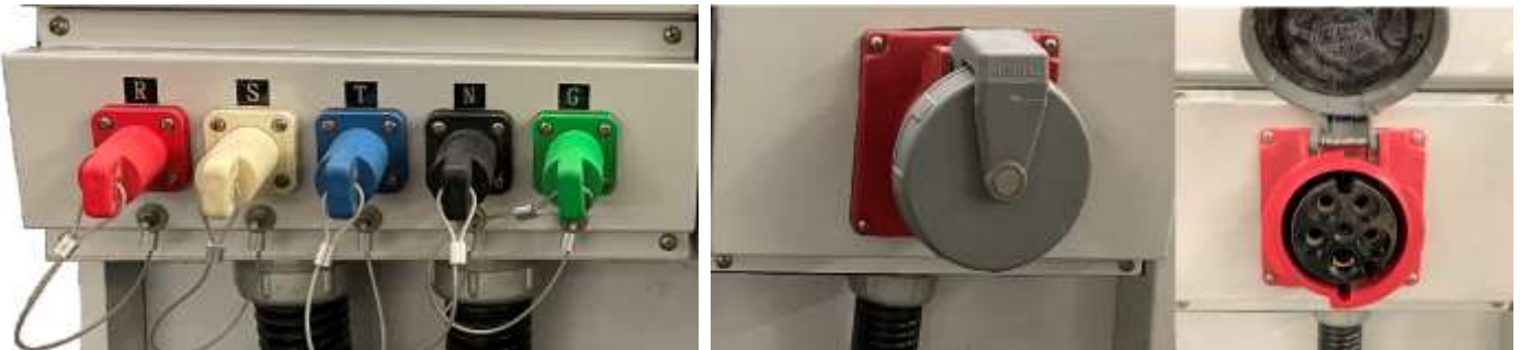
Figure 3.7.1- Additional Power Supply
